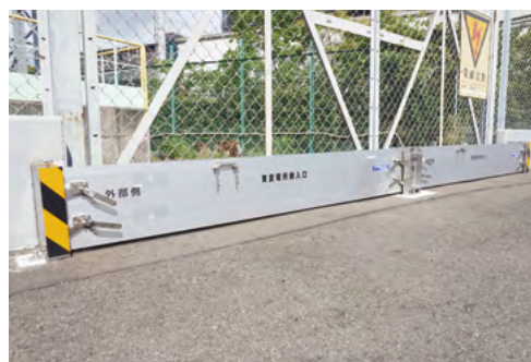
Water barriers installed as a measure against flood damage from heavy rains, etc.
