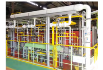
Steel heat treatment furnace with burners installed
