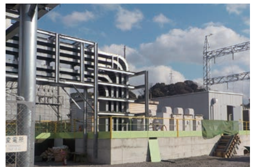
▲ Liquefaction measures: Redesigned in-plant transformer substation
