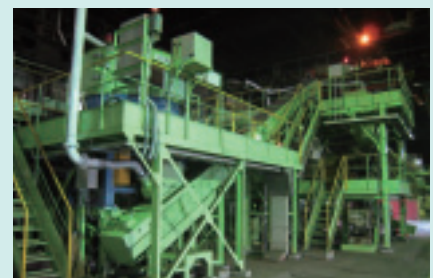
Nickel recycling briquette facility
